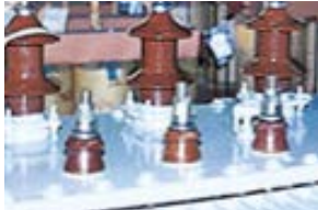
HV bushing with terminal connectors
