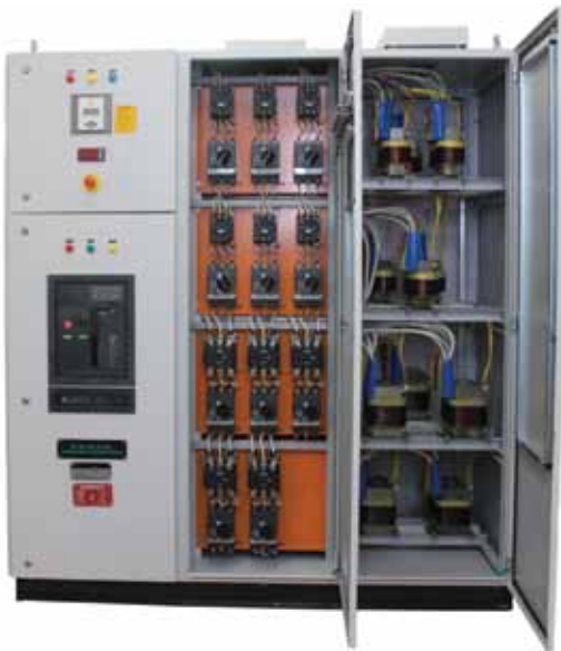
Detuned filter APFC panel
