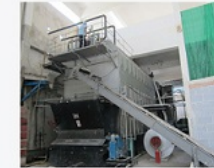
10Ton/h Wood Chips Fired Boiler in Ukraine
