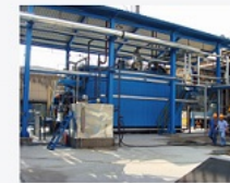
20Ton/h Gas Fired Boiler in Kuwait
