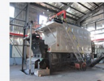
6Ton/h Coal Fired Boiler in Sri Lanka
