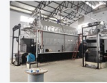
4Ton/h & 12Ton/h Coal Boiler in Pakistan
