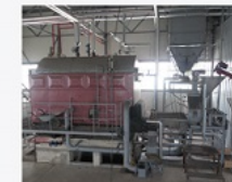
2.5Ton/h Oat Hulls Fired Boiler in Serbia
