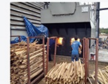
6Ton/h Wood Fired Boiler in Thailand
