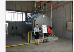
4Ton/h Oil&Gas Dual Fuel Boiler in Myanmar
