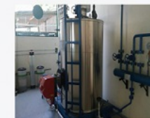
500kg/h Diesel Fired boiler in Indonesia
