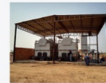
3Ton/h Wood Fired Boiler in Angola
