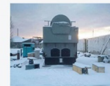
4Ton/h Wood Fired boiler in Mongolia
