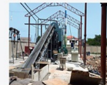
2Ton/h Biomass Fired boiler in Ghana
