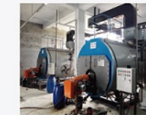
2Ton/h Heavy Oil Fired Boiler in Bangladesh
