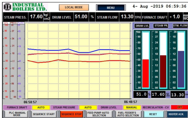
SCADA HMI Display
