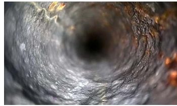
Real life problem 2 Corrosion of Piping
